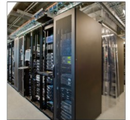
Server towers with racks
